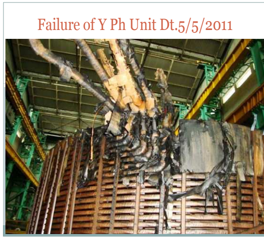
Figure 4: The failed winding top layer
