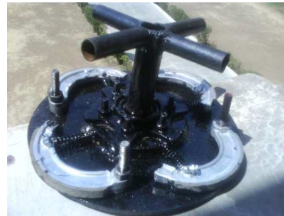
Figure 2.3 Existing Lock Plate which is failing.
