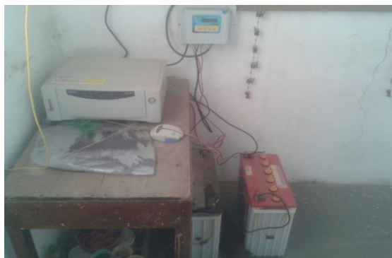
Fig.6: SOLARCON Unit with Battery & Inverter
