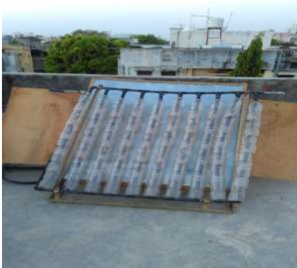
Image: Solar Water Heater
