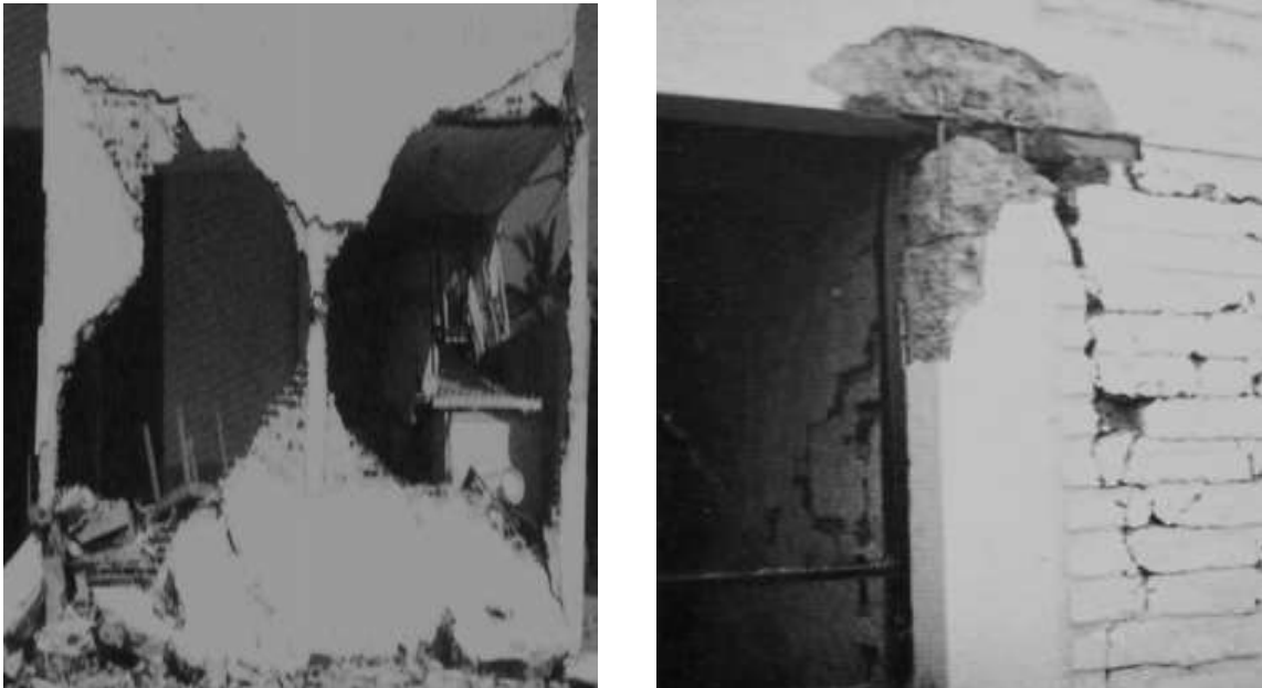
Figure 8. Damage to confined masonry buildings in the 1985 Lolleo, Chile earthquake 1
