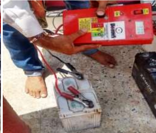
Testing of Battery under Load
