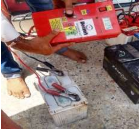
Testing of Battery without load
