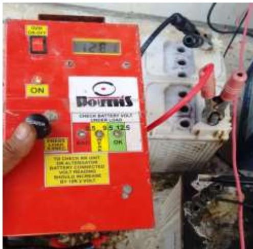
Testing of Battery without load
