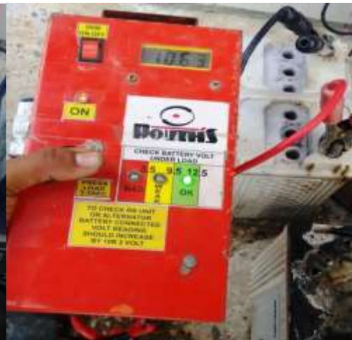
Testing of Battery Under Load
