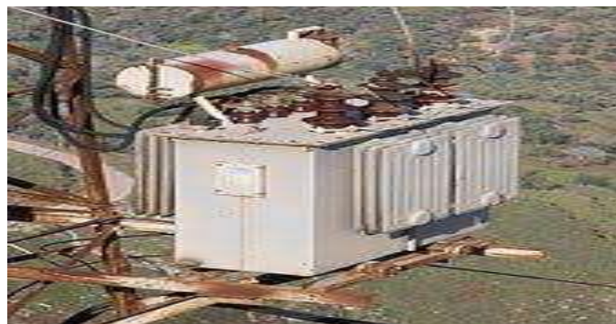
Fig 3: Transformer of 630KV
